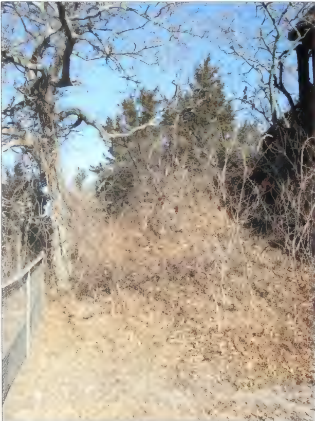
Figure 3.36. View looking northwest at engineered slope to rear of Battery Granger. Between Hudson Drive and the battery, a chain-link fence (left) and signage have been erected to warn visitors of potentially hazardous conditions (Olmsted Center, January 2009).
